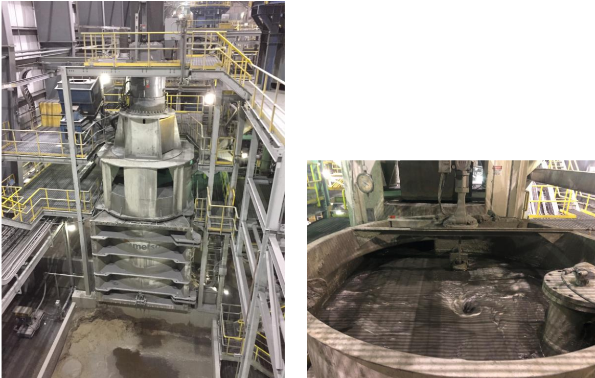
Figure 7 – Vertimill and Separating Tank
